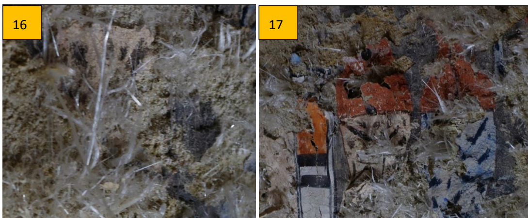
Photo 16-17 Crystallization of salts on the surface of the bedrock
