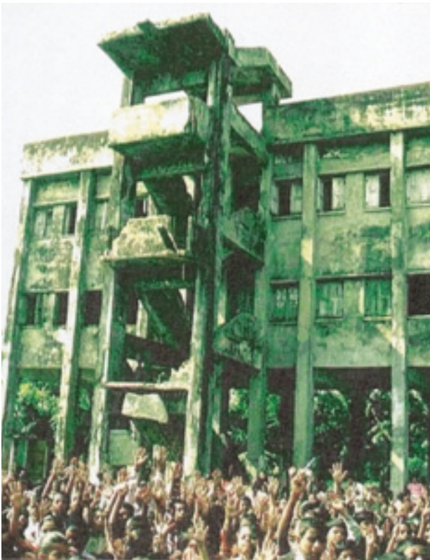
Photo 1 Cyclone shelter made of corroded reinforced concrete; it is used as an elementary school building for dual lessons
