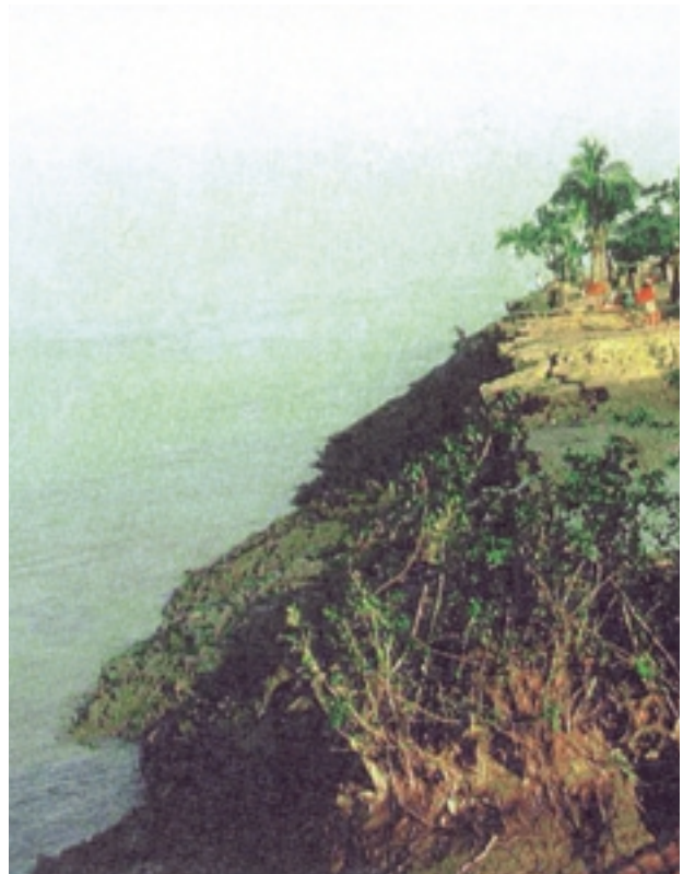
Photo 2 Severely eroded coast
